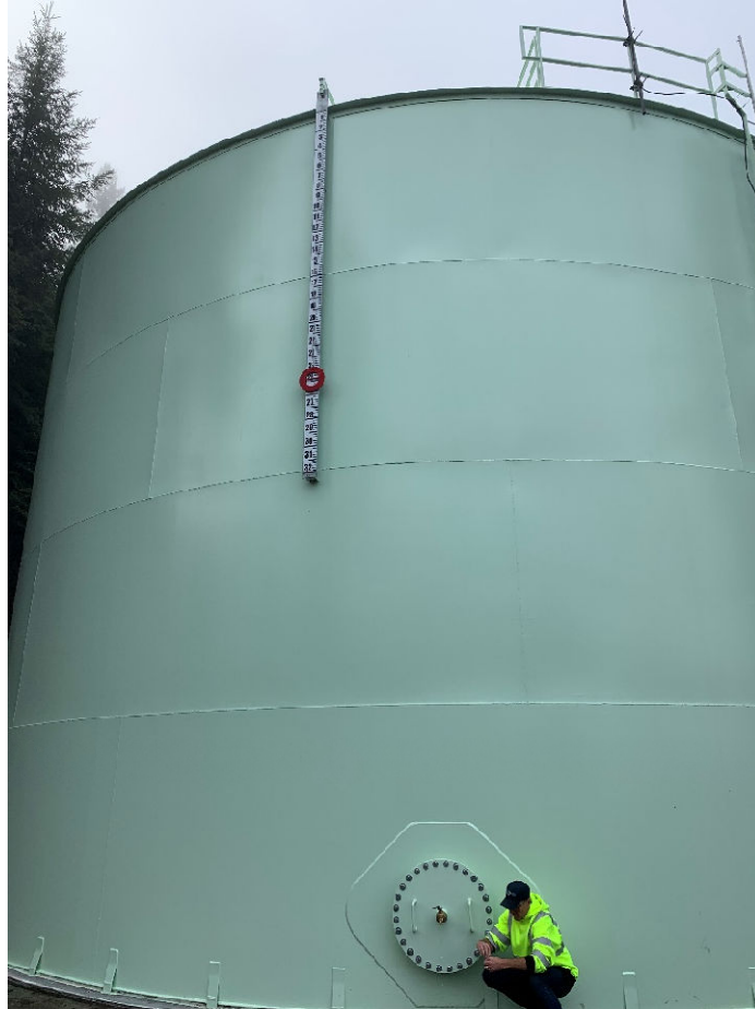
Figure 2: Picture of the District's actual Brier Lane Tank taken after the rehabilitation contractors completed the rehabilitation project. In the picture you can see that the tank is filled to 23 feet and that a District operator is collecting water quality samples for contamination testing.
