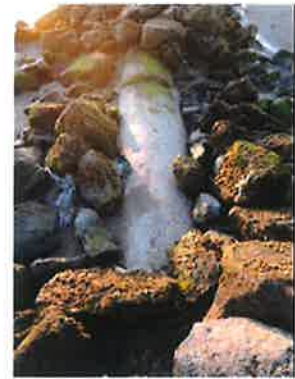
Figure 3: Example Damage to the Existing Near Shore Pipeline, Since Repaired
