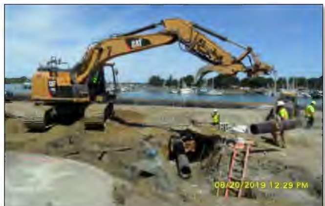
SHN provided construction management services on the City of Eureka's Waterfront Drive project in 2019.
