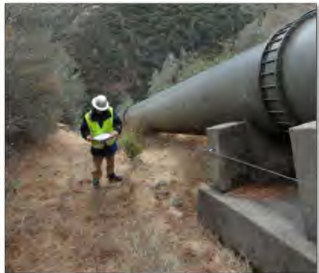
SHN's Geosciences group is accustomed to working in remote and rugged conditions.
