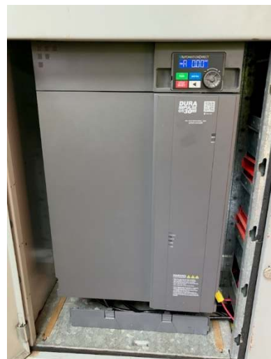
Figure 2: This figure shows the newly installed Variable Frequency Drive (VFD) used to modulate flow and improve energy efficiency of the system
