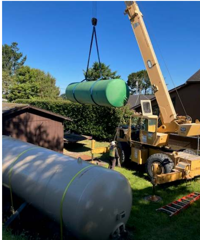
Figure 2: New hydro-pneumatic tank in place at the Donna Drive tank site while old hydro-pneumatic tank is being lifted over a building to be hauled away for recycling.
