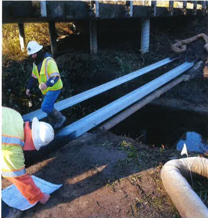
Figure 1: HCSO Construction crew working to place armoring treatment over aerial crossing over Martin Slough.
